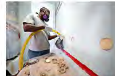
Workers like this one putting insulation into a wall will help transform public and private sector buildings through energy upgrades. Credit: Dennis Schroeder, NREL
